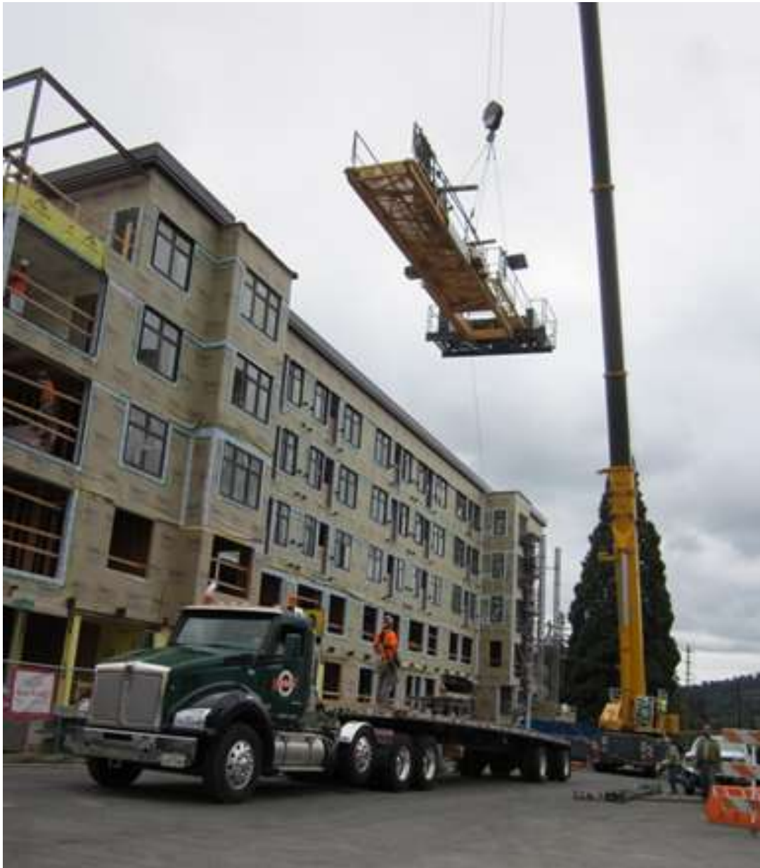
The rear main section of the tower crane is lowered onto a waiting truck
