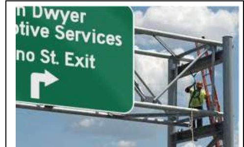
A worker puts the finishing touches on the new Tenino Street Exit sign.
